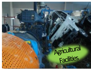
A drainage facility in Soma City
