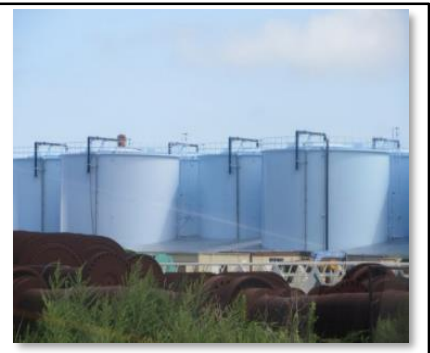
Tanks at F1NPS Current situation of treated water at F1NPS (as of 25 June, 2020) Number of tanks: 1,006 tanks Storage volume in the tanks approx. 1.21 million m 3
