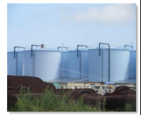
Tanks at F1NPS
