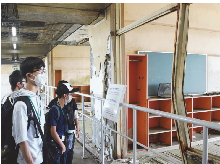
A classroom hit by the tsunami. The remaining steel frame is bent.
