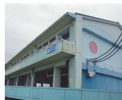
The school building is a two-story reinforced concrete structure with an illustration of the sun and the sea on the wall. (Right side of the photo)
